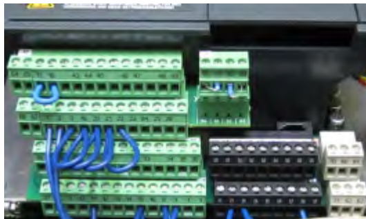
Peripheral board terminals
