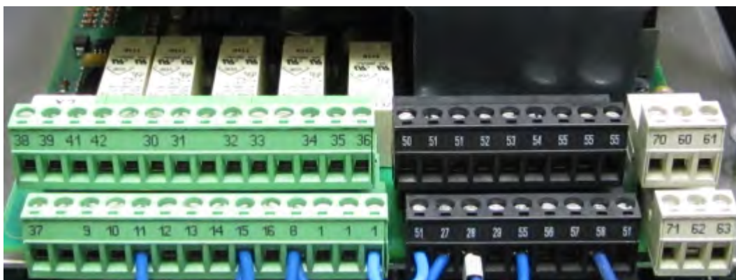
Figure 8-13 Control cable terminals
