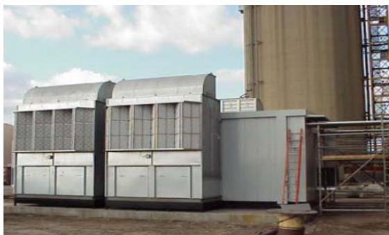
Figure 8 Installation with Air-to-Air Heat Exchangers and two drives in the building
