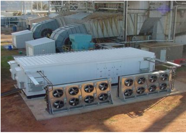
Example of installation with W32 option: there are 2 WC drives in the building
